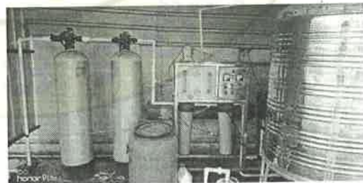
Reverse Osmosis Plant
